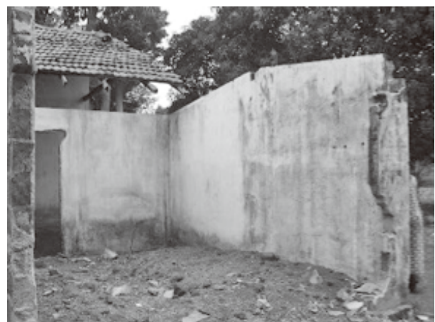
Destroyed house of Sivarajani.
