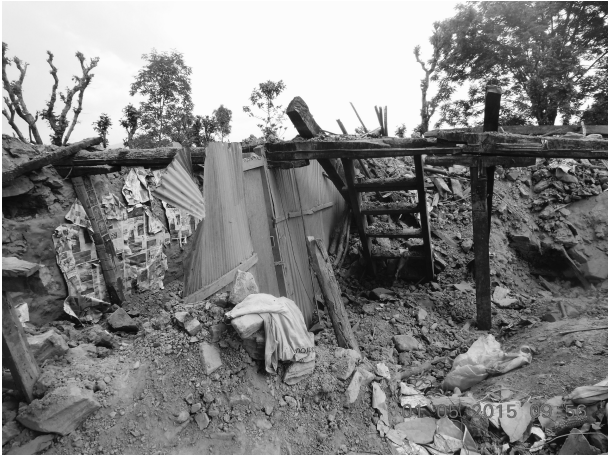
Destroyed house in Sindhupalchowk, Nepal. Photo by BBP-Pariwar.
